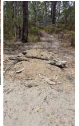
Erosion taking place
