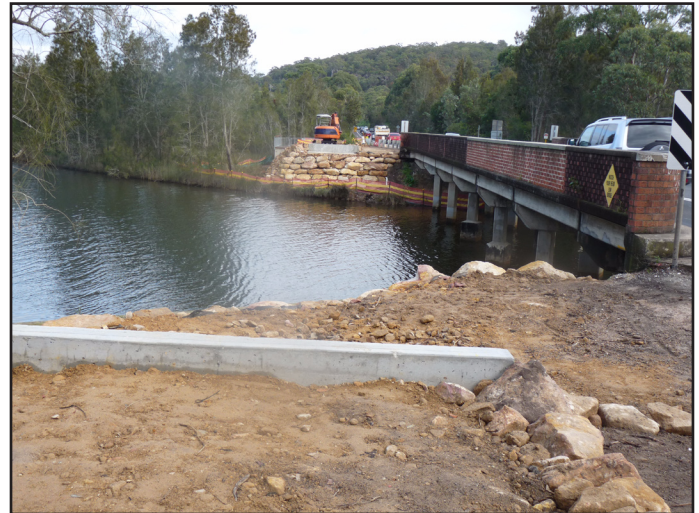
The approaches to the footbridge on each side of Deep Creek seem to be ready for the span to be fitted.
